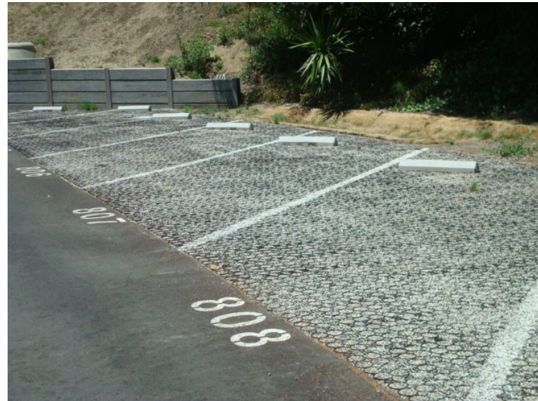
Permeable paving allows stormwater to filter through the surface of parking lots, improving water quality and reducing runoff handled by storm drains
