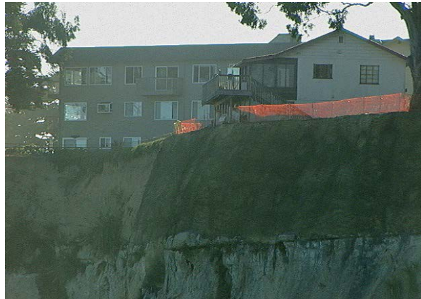
Property on bluffs impacted by erosion and landslides
